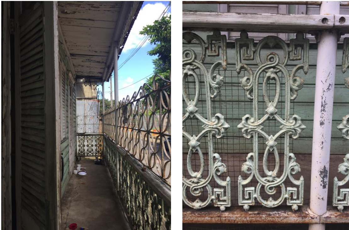
Figure 5: Views of Casa Vigil's porch (looking north) and cast iron railings, 2017. (YMCR)
